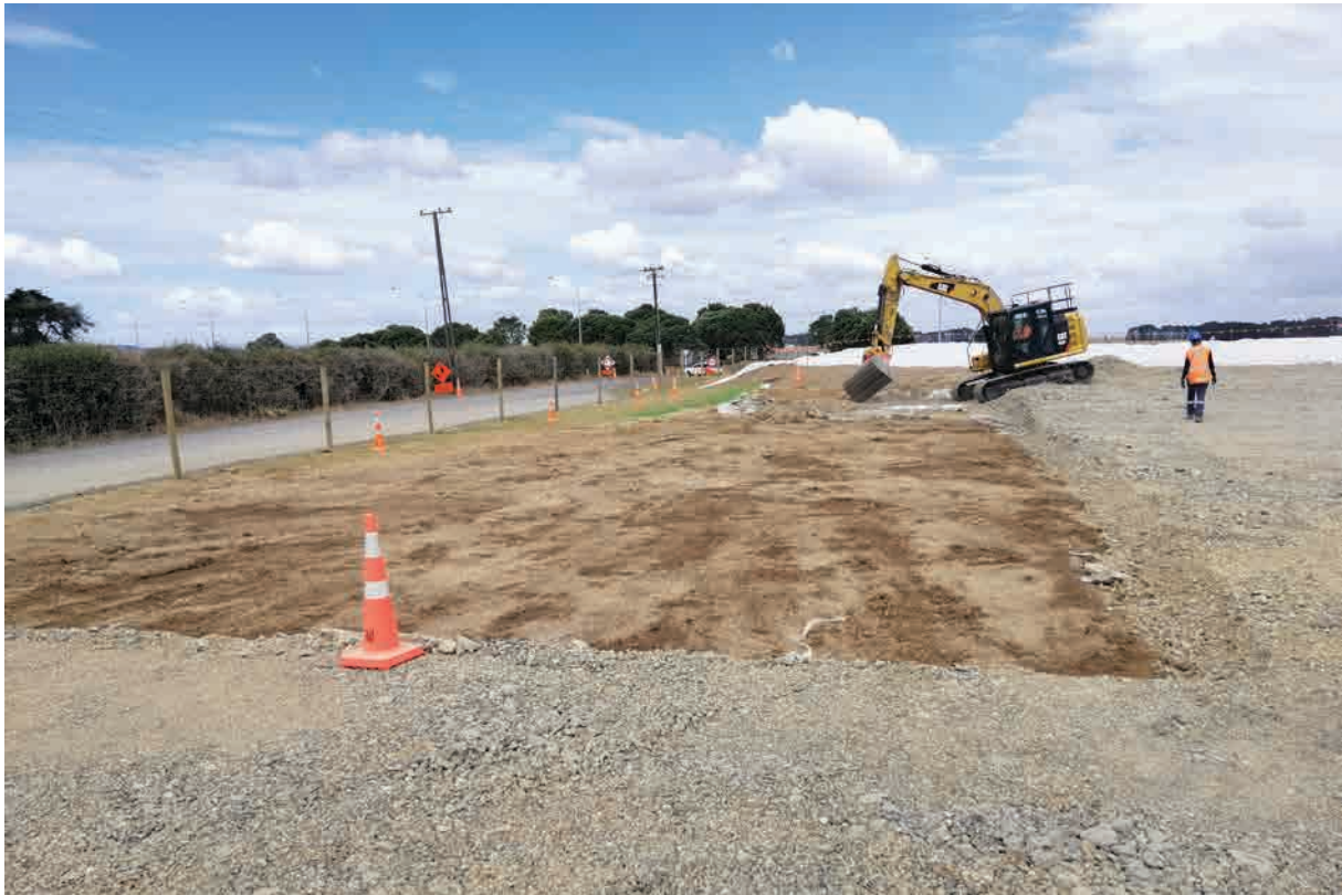
Figure 5. View south of silt pond being built next to Orrs Road, with metal laid for the laydown.
