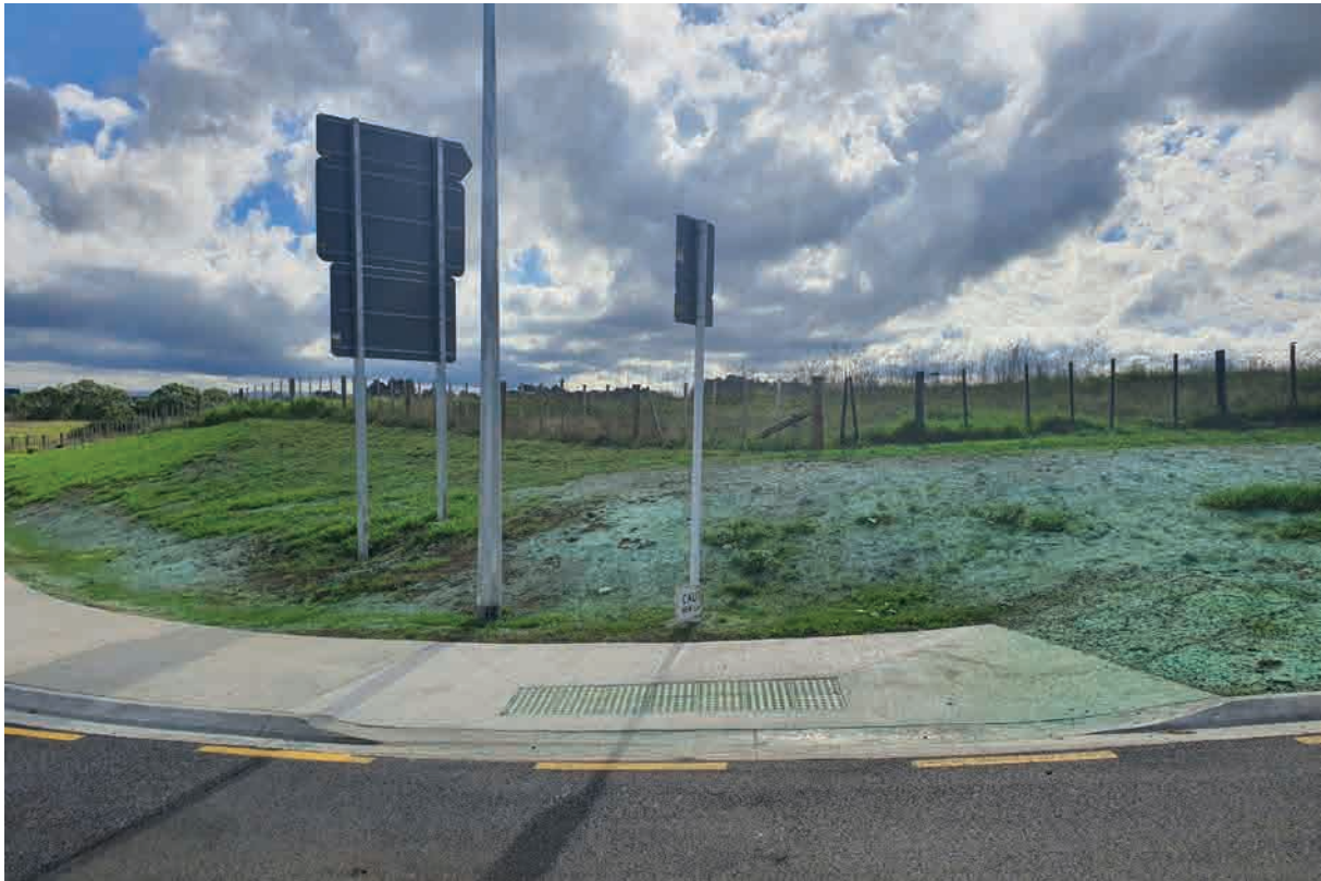
Figure 8. Works near Papāhīnau Chapel – the recorded location is in the paddock in the background.
